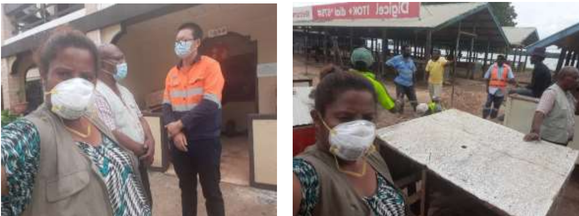
Photos 13-14. PNG Water doing piping for the hand washing basins at the Kavieng Market as part of PCC measures in New Ireland Province
